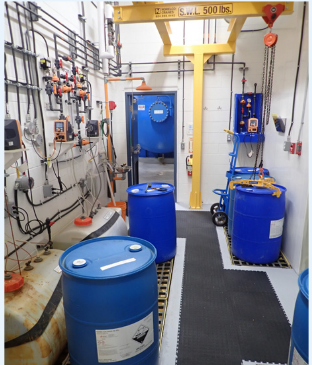
Picture 9 – New crane to move 45-gallon chemical drums.
