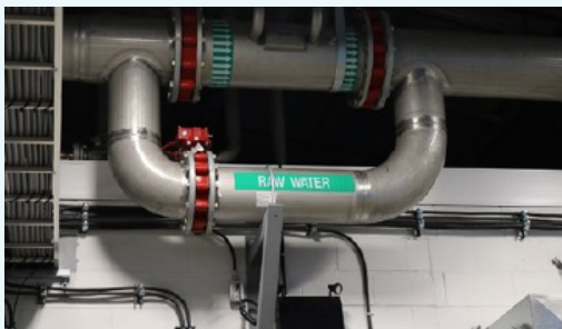
Picture 6 – Ozone injector into raw water before filtering
