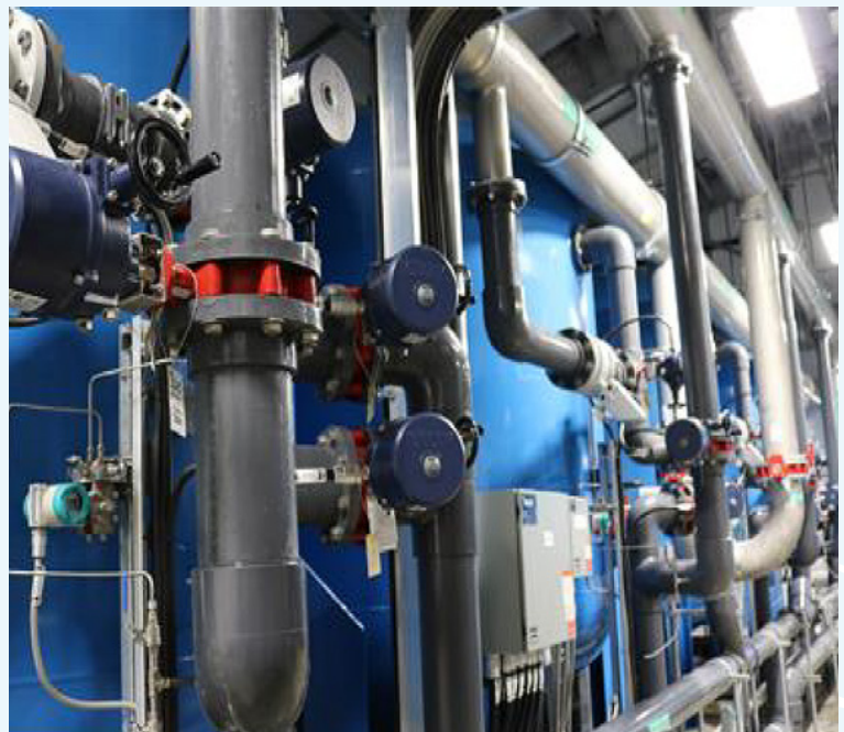
Picture 8 – Adedge E33 filter tanks to remove arsenic
