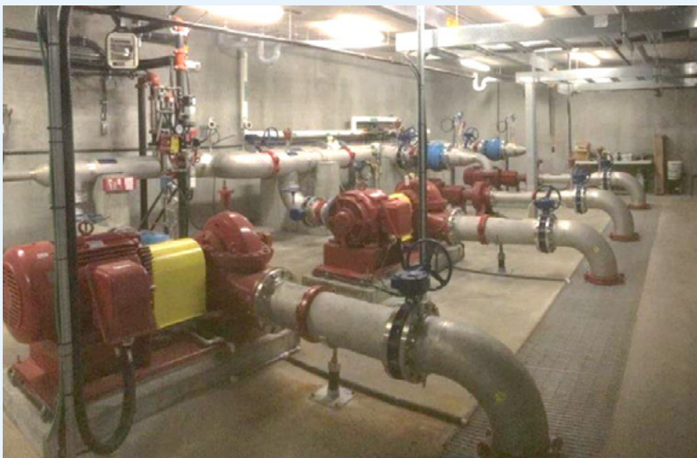
Picture 1 – Booster pump station
