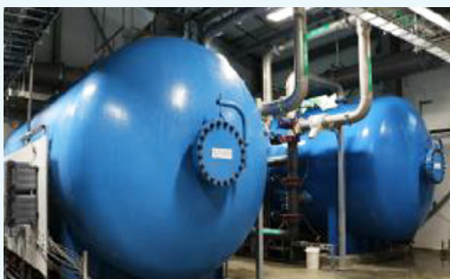
Picture 7 – Greensand filter tanks to remove manganese
