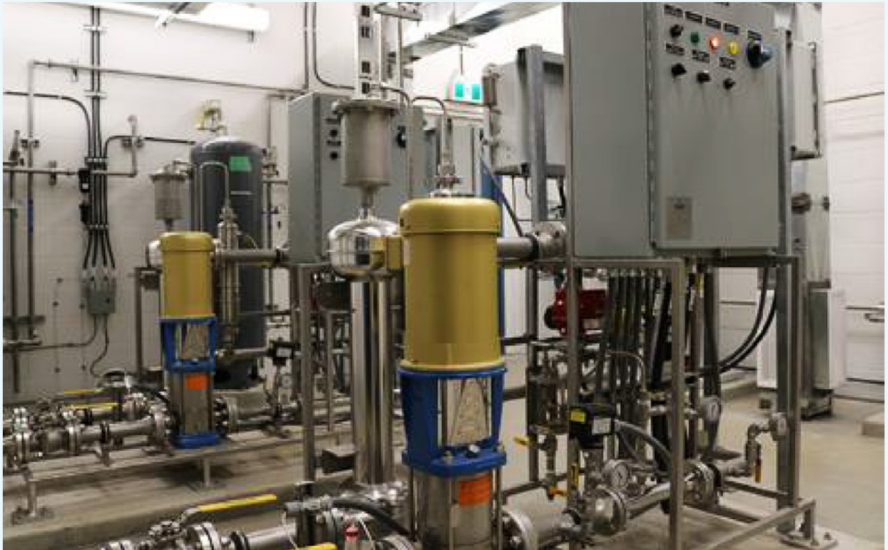
Picture 5 - Water Treatment Plant Ozone System
