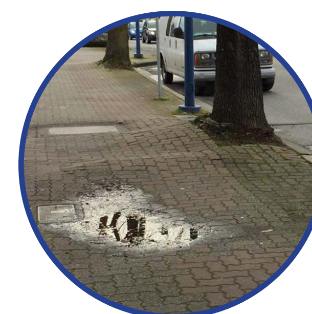
POOR DRAINAGE CONDITIONS
