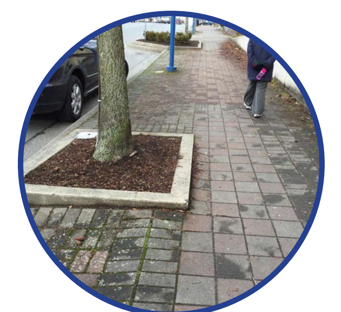
TRIP HAZARDS ON SIDEWALKS
