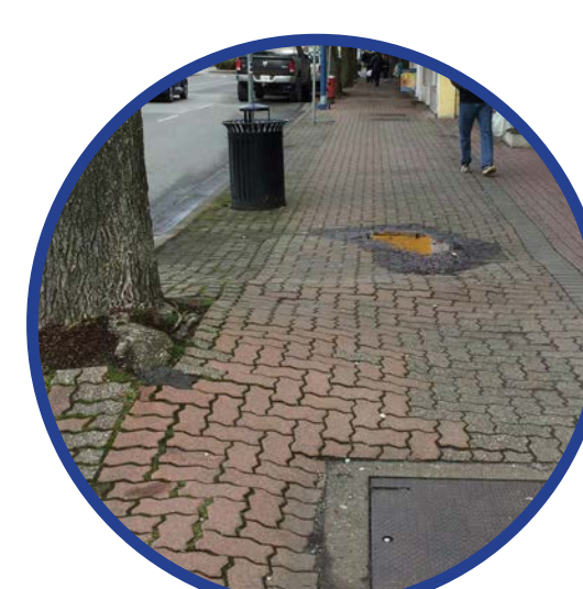
POOR SIDEWALK CONDITIONS
