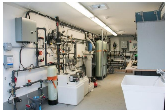
Figure 12: Inside the Mobile Trailer
