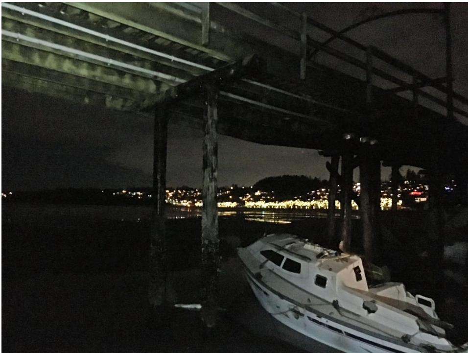
Photo 7: Boat debris lodged between pile bents
