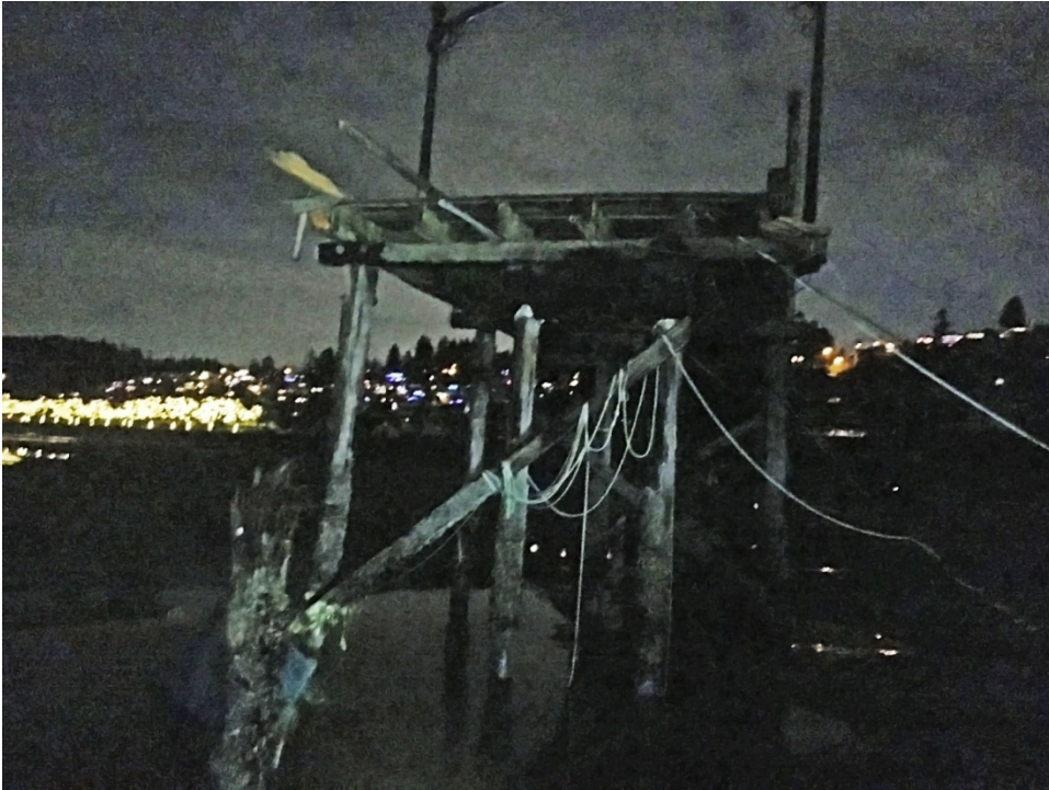
Photo 3: Failed section of Pier between Bent No. 33 to 44
