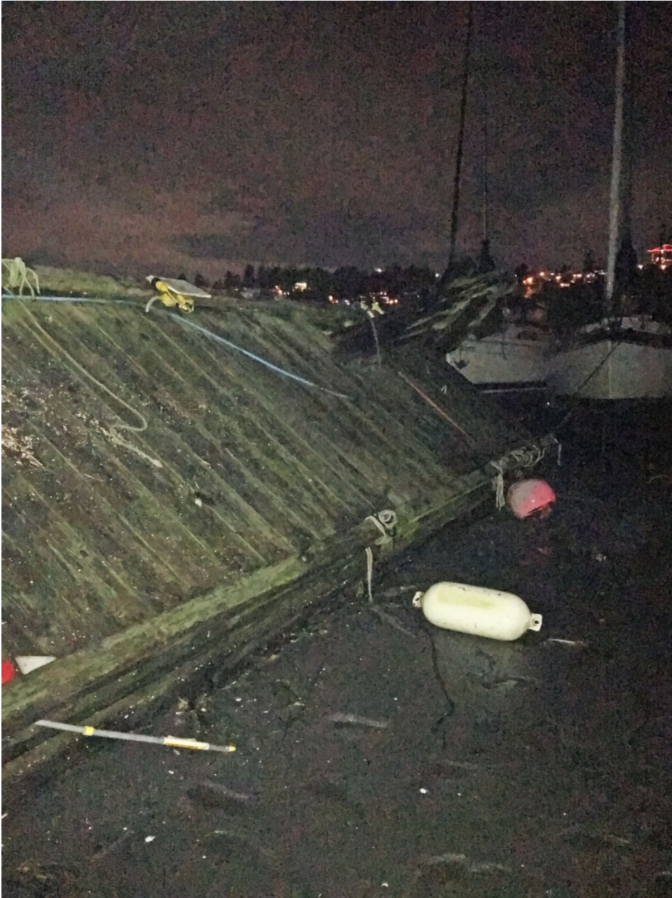
Photo 4: Failed section of West Marina Float
