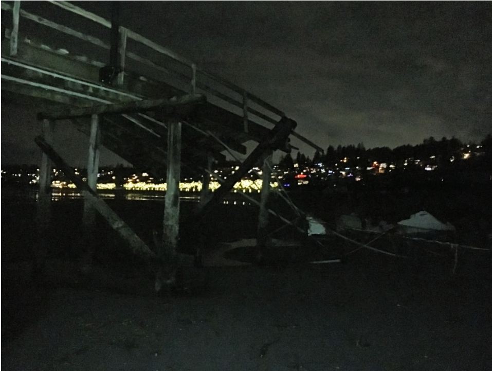
Photo 1: Failed section of Pier between Bent No. 33 to 44
