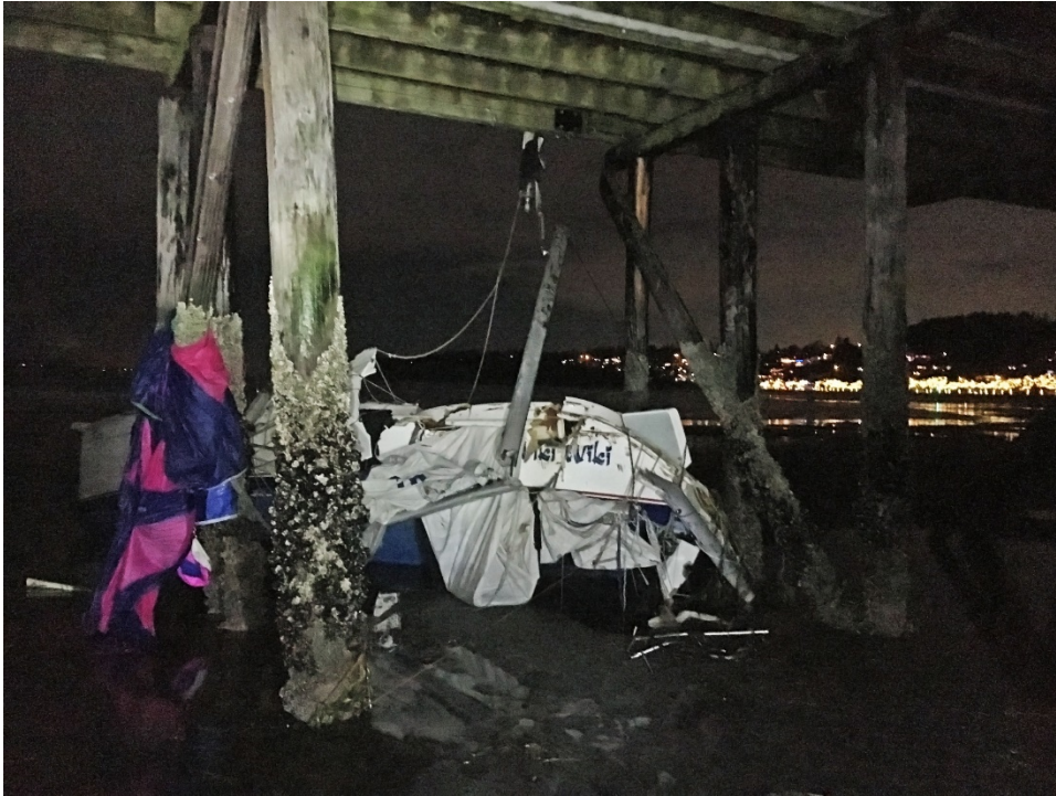
Photo 6: Boat debris lodged between pile bents
