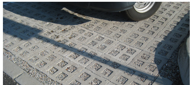
Guideline c: Permeable pavers Image: Center for Watershed Protection Inc.
