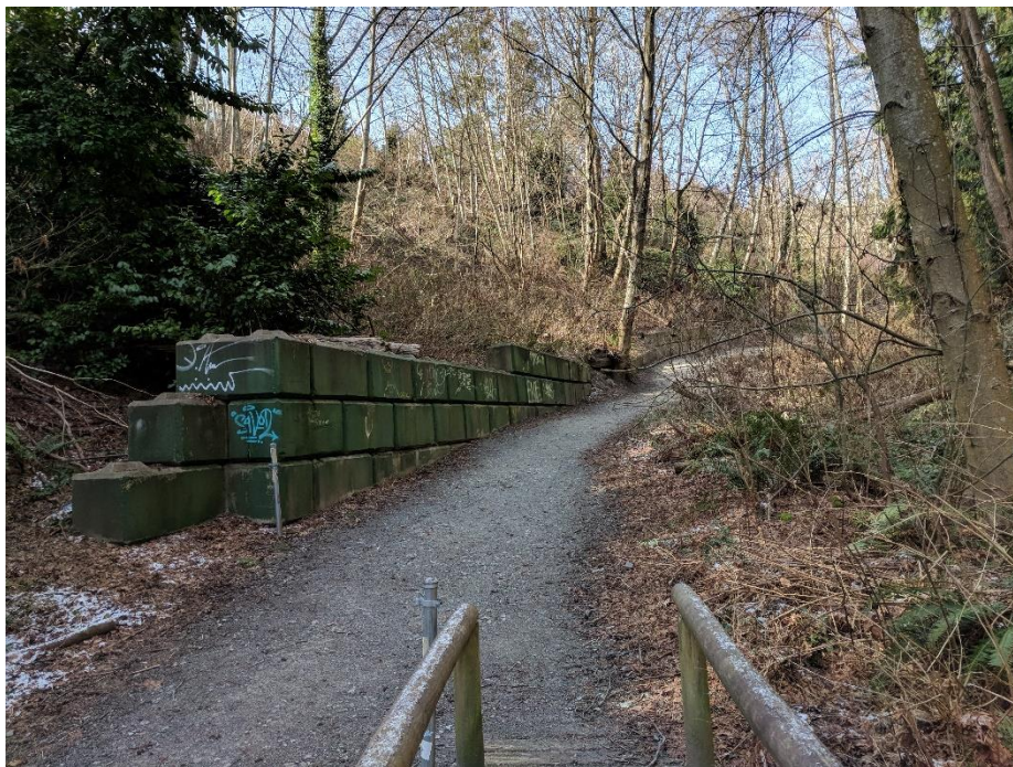
Photo 9 Duprez Ravine – Current Condition of Slope at 14517 Magdalen Avenue
