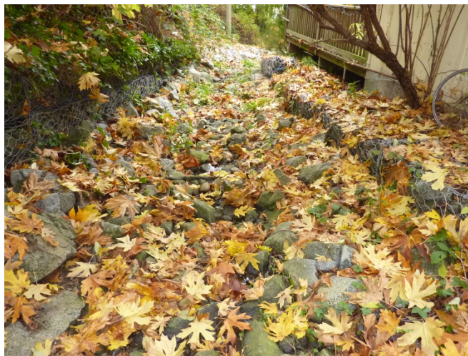
Photo 10 Everall Ravine – Rip Rap Armour and Gabion Wall Lined Channel above Inlet Structure
