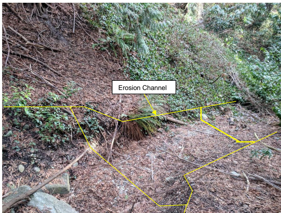
Photo 14 Everall Ravine West Brach – Erosion Channel below Pipe (Looking downslope, 3 m below end of CSP)
