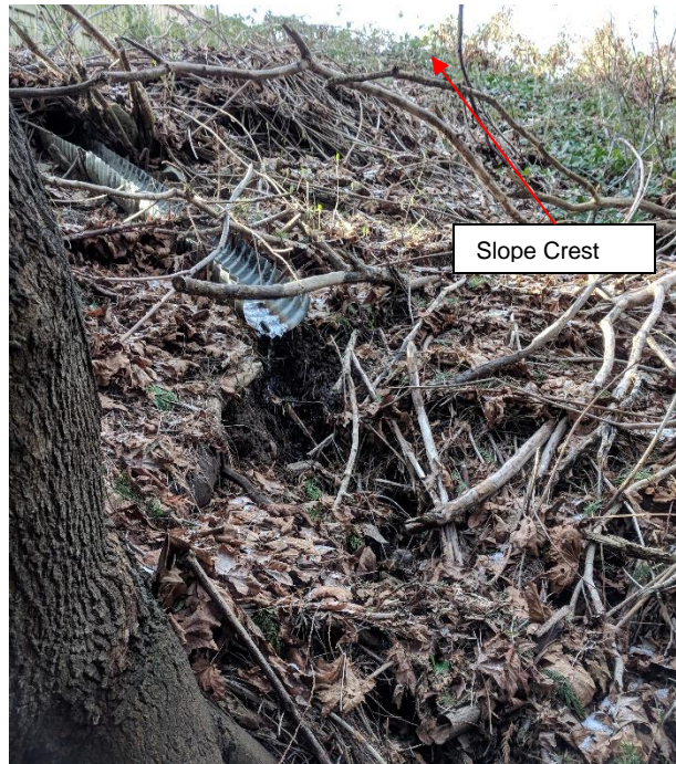
Photo 13 Everall Ravine West Branch – CSP Pipe near Crest
