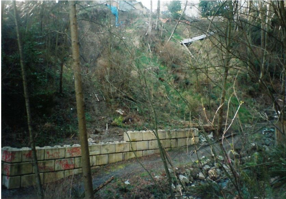
Photo 8 Duprez Ravine – Landslide at Crest of Slope at 14517 Magdalen Avenue in 2000
