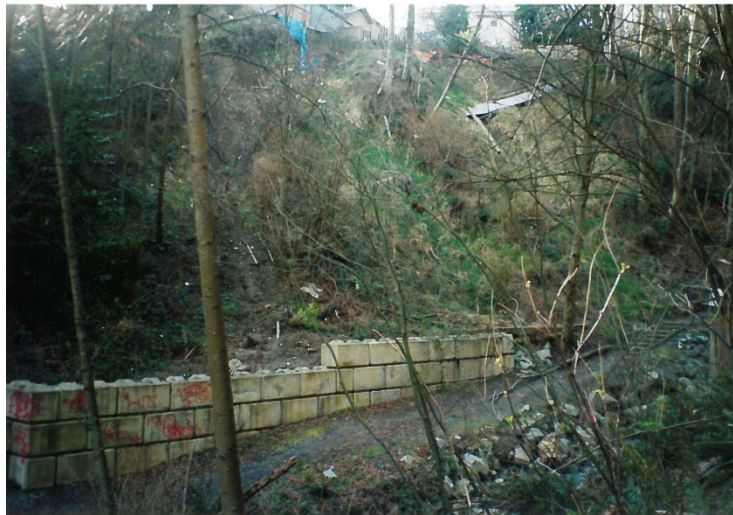
Photo 4 – Duprez Ravine– Landslide at Crest of Slope at 14517 Magdalen Avenue in 2000
