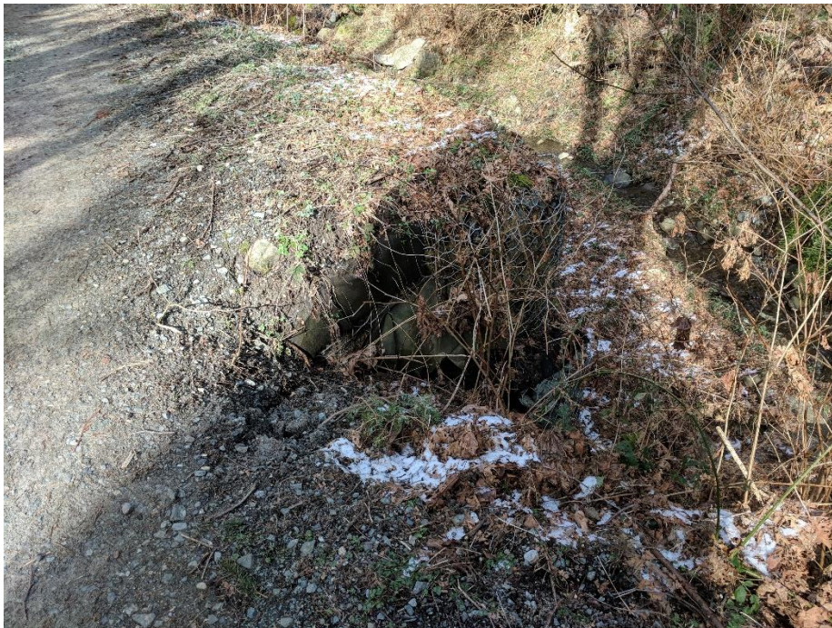
Photo 7 Duprez Ravine – Sinkhole Behind Gabion Wall at base of 14517
