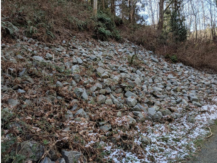
Photo 6 Duprez Ravine – Current Condition of Repaired Slide at Inlet Structure
