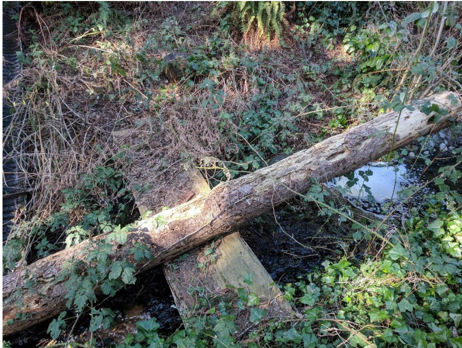
Photo 4 Collingwood Ravine – Foot Bridge Collecting Debris
