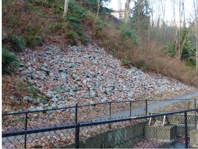
Photo 3 Duprez Ravine – Current Condition of Repaired Slide at Inlet Structure
