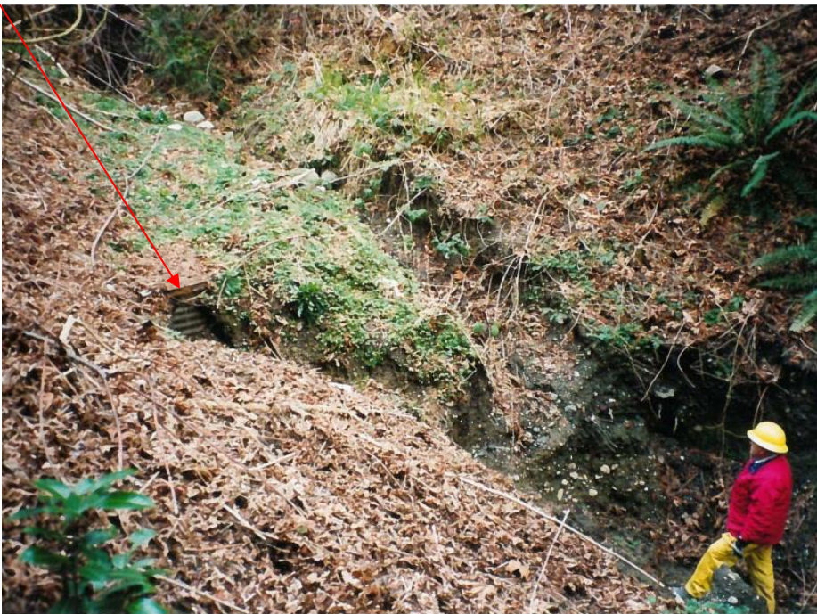
Photo 16 Everall Ravine – Creek Channel Damage in 2002
