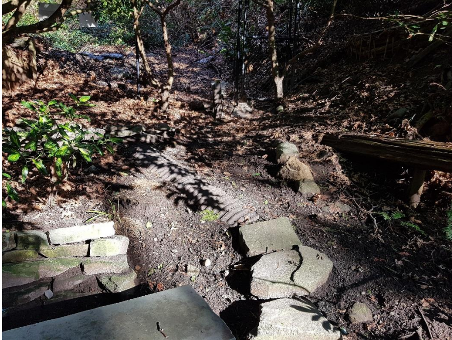
Photo 17 Everall Ravine – Storm Water Pipe Exposed in Ravine Floor
