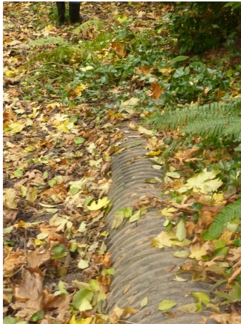
Photo 8 Everall Ravine – Storm Water Pipe Exposed in Ravine Floor
