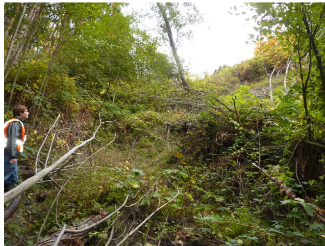
Photo 2 Lower Coldicott Ravine - Recent Landslide on West Ravine Slope Below Private Properties
