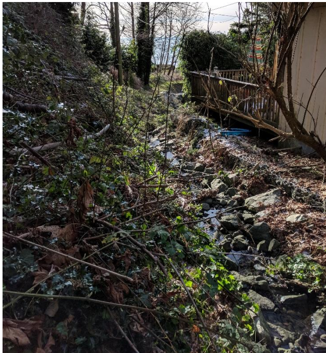
Photo 20 Everall Ravine – Gabion and Rip Rap Armour Lined Channel above Inlet Structure
