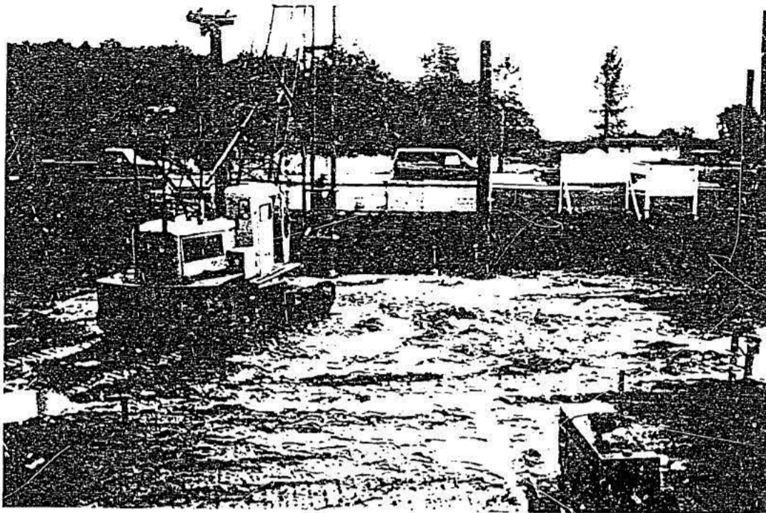
9. Looking towards the south showing condition of excavation base after a heavy rainfall. Slope cut height along south excavation wall was approximately 5 to 6 feet.
