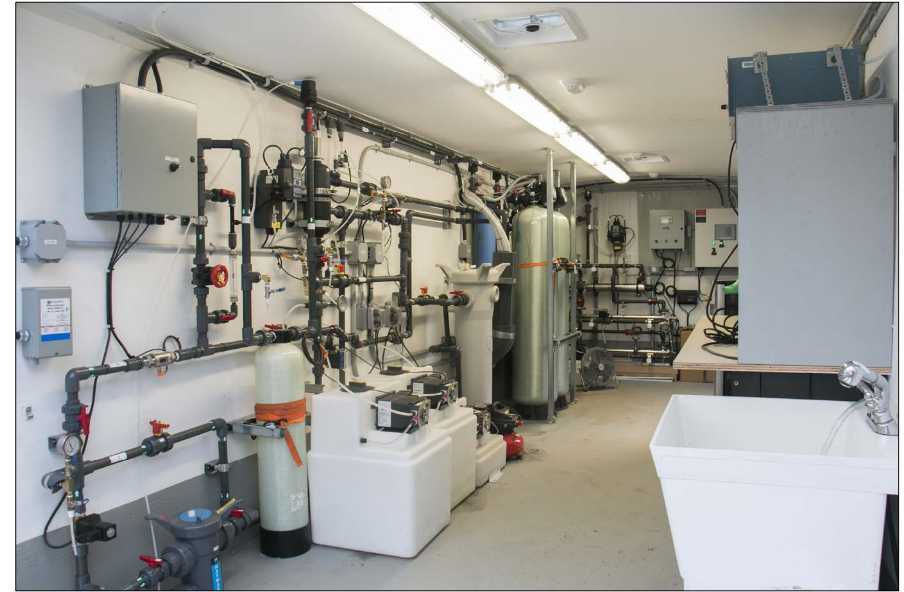
Figure 1 RES'EAU-WaterNET mobile drinking water treatment pilot plant.
