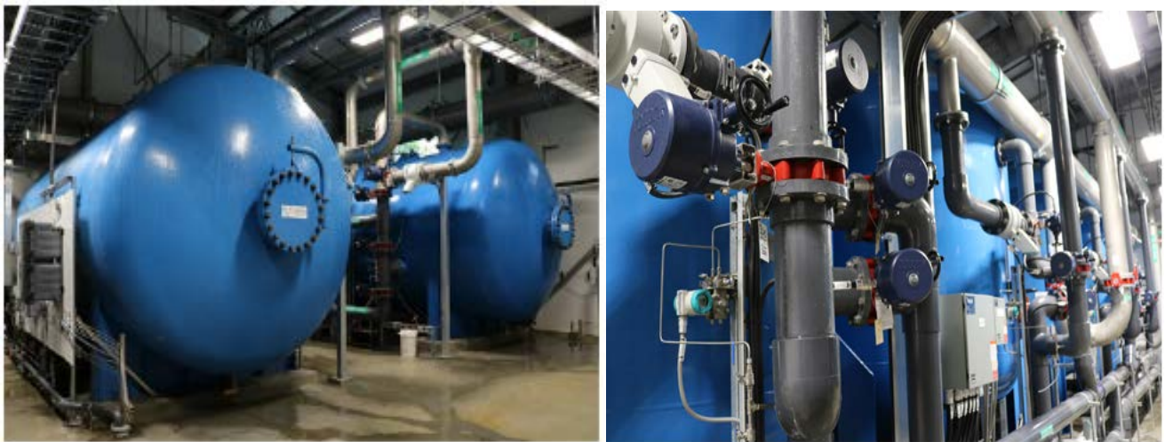
Figure-9, The newly constructed White Rock Water Treatment Plant
