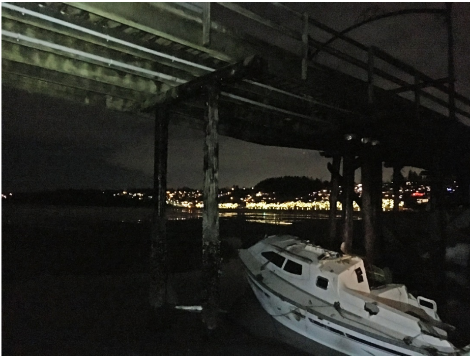
Photo 7: Boat debris lodged between pile bents
