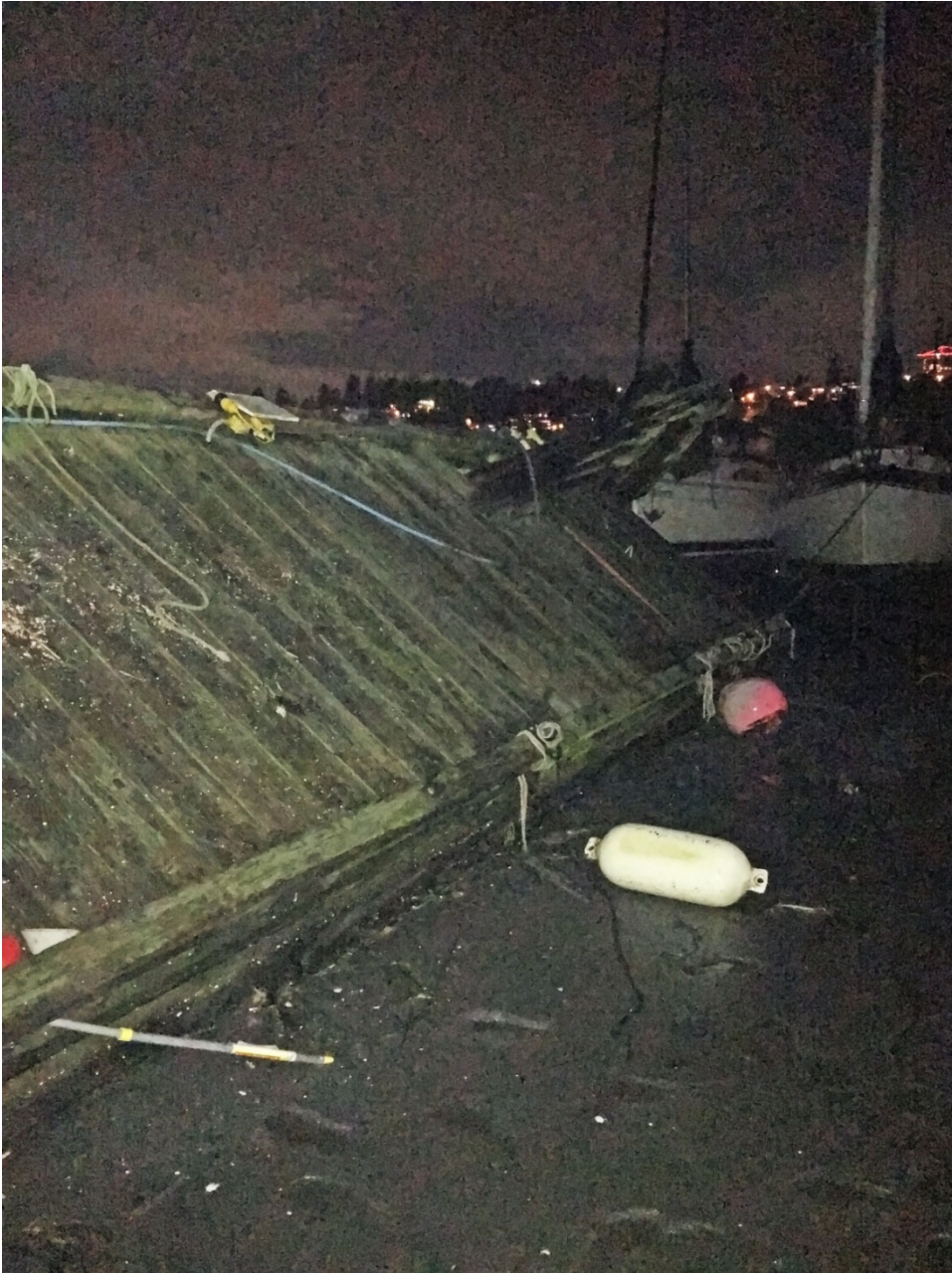
Photo 4: Failed section of West Marina Float
