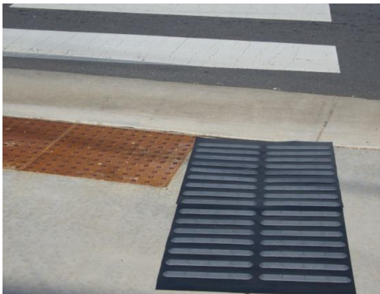
Figure 3. Photo of a guidance surface with raised bars perpendicular to the direction of travel across the crosswalk (Bentzen et al. 2017).
