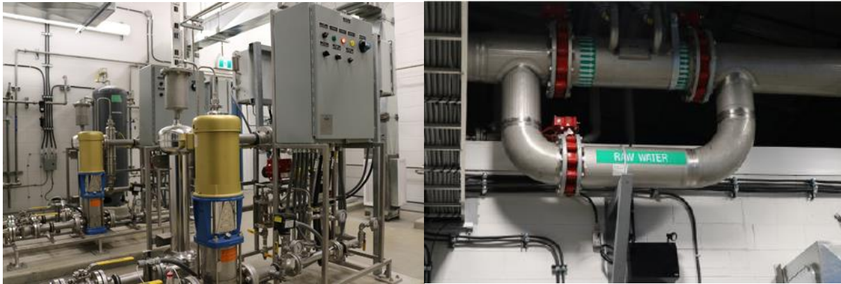
Figure-8, Water Treatment Plant Ozone System
