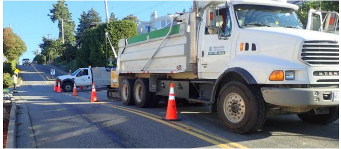
Figure-11, Oxford at Prospect Avenue and McDonald Avenue tie-ins to 200mm watermain on Oxford Street
