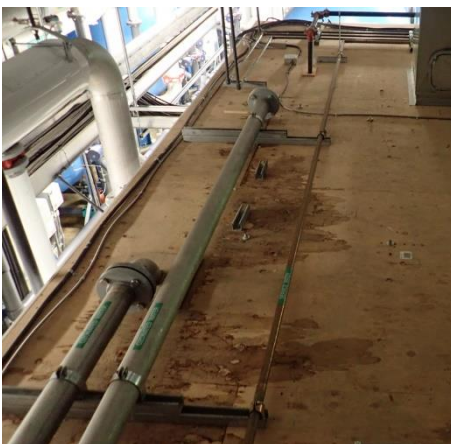
Figure 12 - Pipe before insulation showing condensation on the wood
