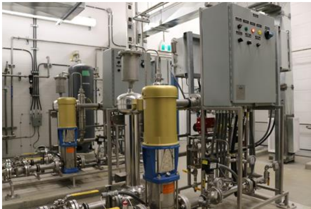
Figure 8 - Water Treatment Plant Ozone System
