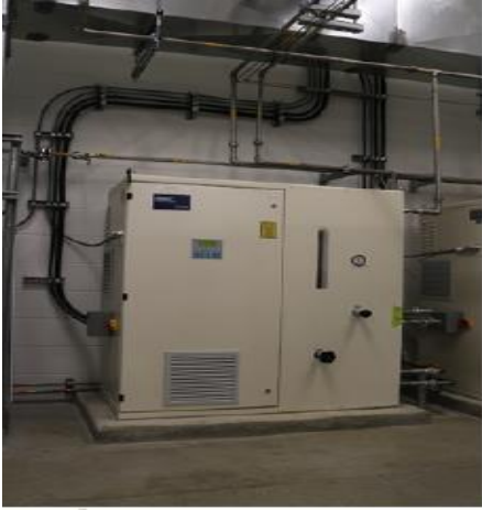
Figure 7 - Water Treatment Plant Equipment
