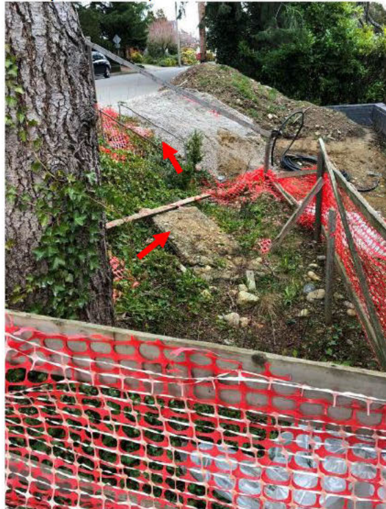
Figure 3. Old stairs and other debris to be removed.
